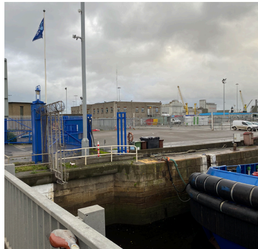
▲ Existing quay wall of Berth 18 in use for tug boats and cruise liners docking
