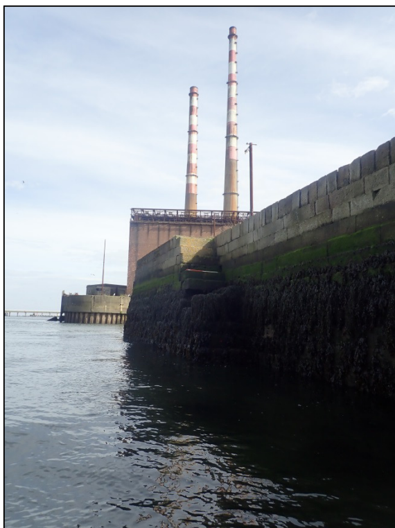
Plate 36: East-facing view of channel side façade of historic pier-head (Feature F02) at entrance to Pigeon House Harbour (1m scale).
