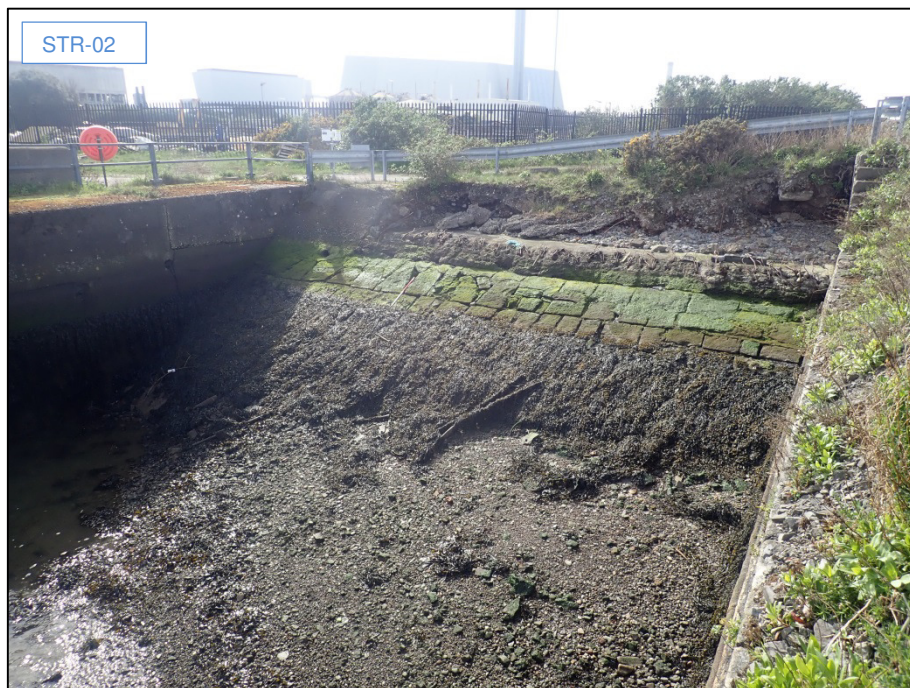
Plate 45: Southwest-facing view of section of angled retaining-wall (STR-02) located at northwest corner of Pigeon House Harbour (modern extent), ITM 720283E, 733836N; STR-02 comprises the remains of a substructure to a boat launch (1m scale).
