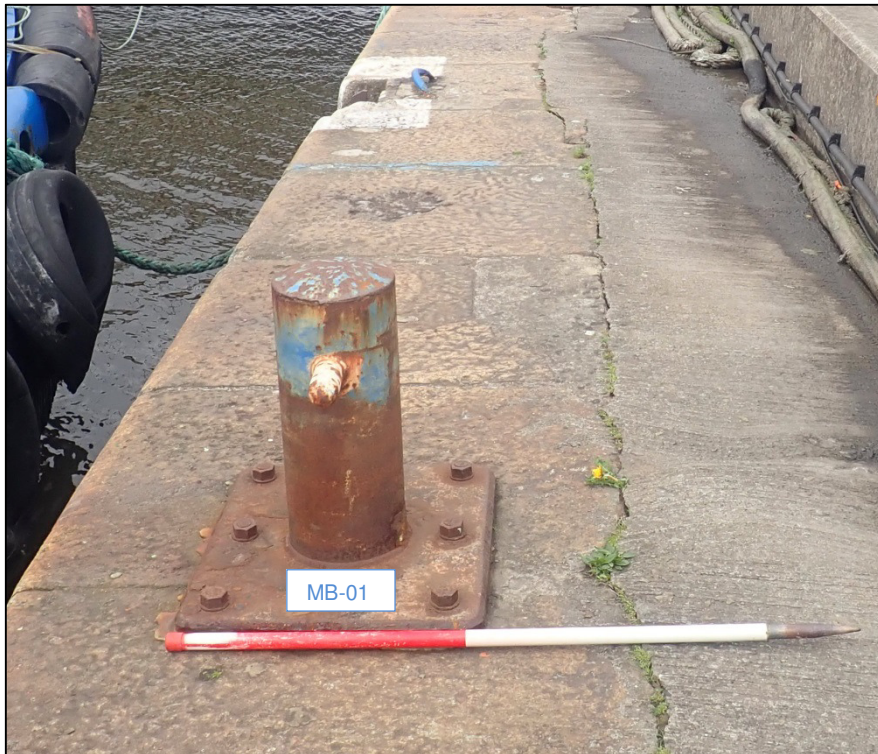
Plate 28: Cast-iron mooring bollard (MB-01) located between mooring hoops MH-01 and MH-02, at ITM 718034E, 734383N (1m scale).
