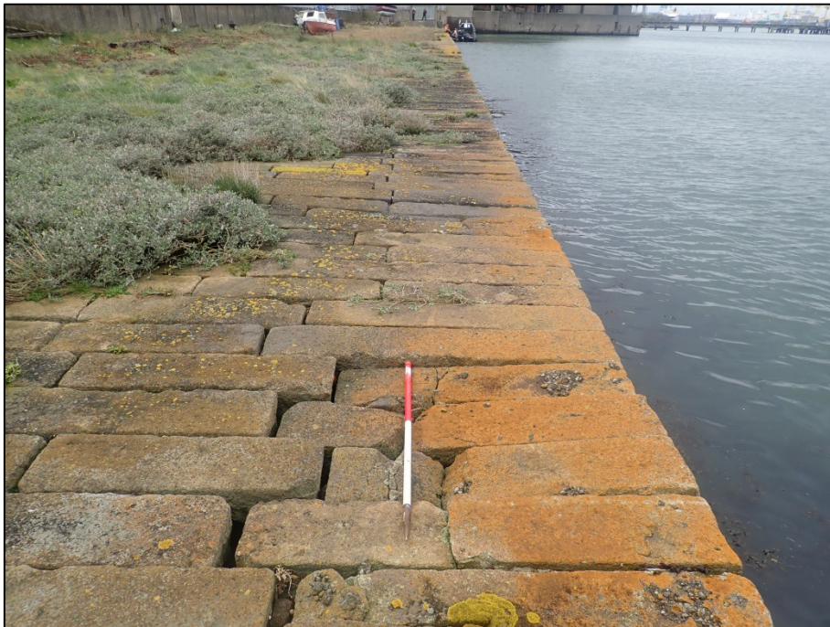
Plate 61: West-facing view of the surface of the sea wall where slumping/separation of masonry has occurred; Survey Area 4; GSW-West (1m scale).
