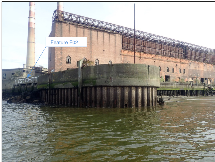
Plate 48: Southeast-facing view of pier-head forming east side of harbour entrance, note presence of original quay-wall behind this structure.
