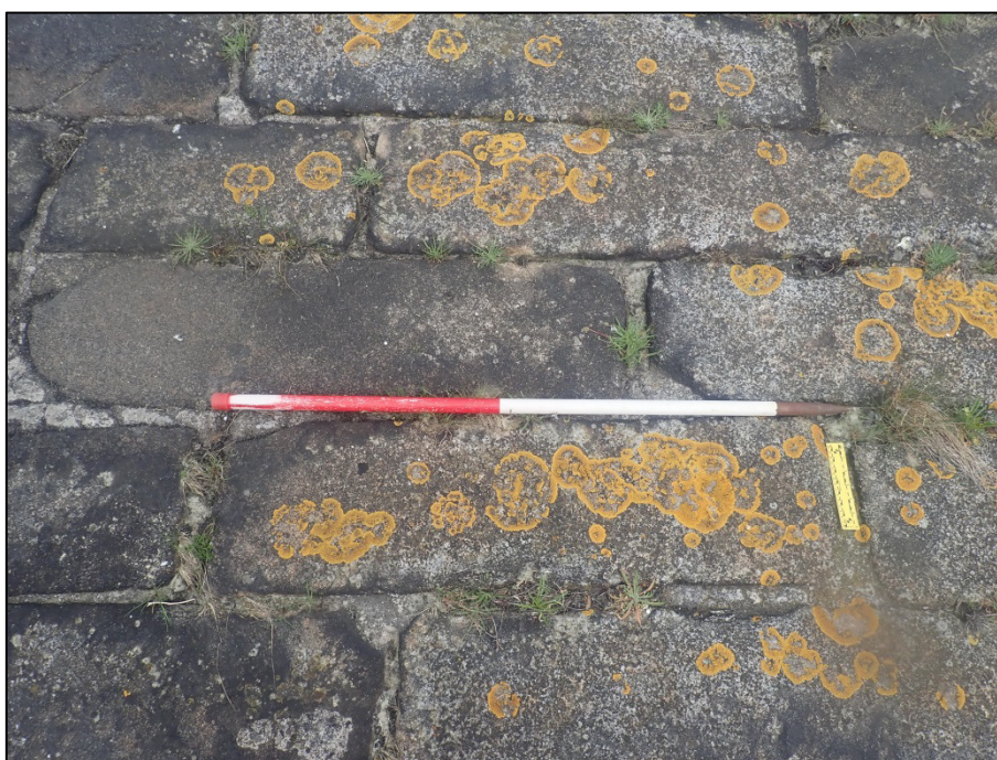
Plate 73: Example shot of deck masonry forming surface of the sea-wall (Survey Area 4; GSW-west 2); repointed using cement (150mm/1m scales).
