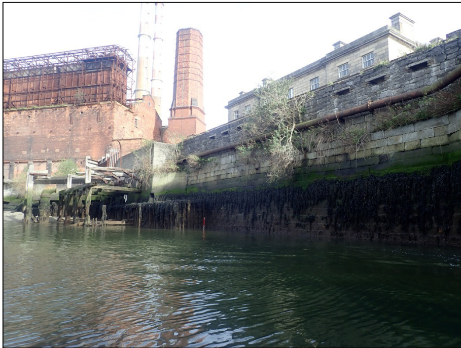
Plate 54: East-facing view of masonry quay that delineates the southeast part of the harbour basin (Feature F03), note underpinning of quay and timber wharf to left of picture (1m scale).
