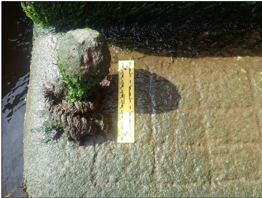
Plate 20: Detail shot showing eroded boat tie-off fitting from RAS-01 (150mm scale).
