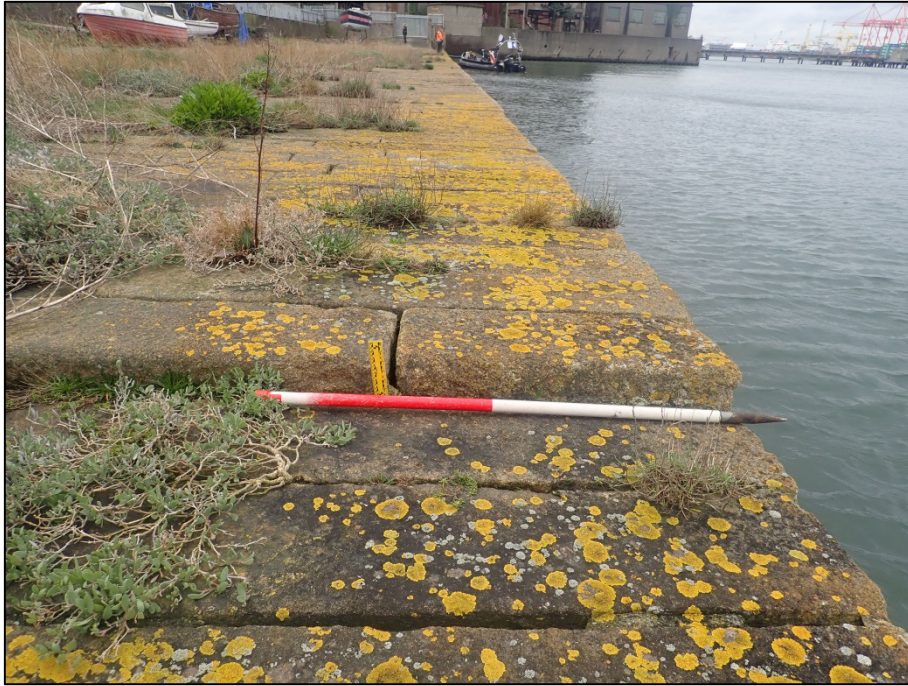
Plate 62: West-facing view of the surface of the sea wall at a point where there is a noticeable drop in the deck-level; Survey Area 4; GSW-West (150mm/1m scales).
