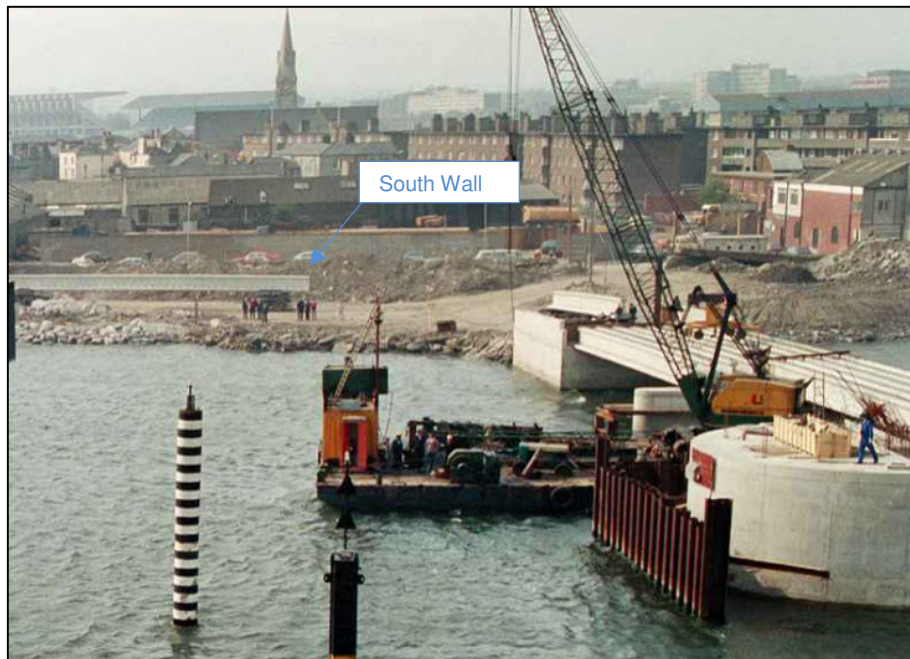
Plate 3: South-facing view of the construction of the East-link Bridge (1983-84) showing reclamation of the foreshore on the south side of the channel [source: Bridges of Dublin, DCC].
