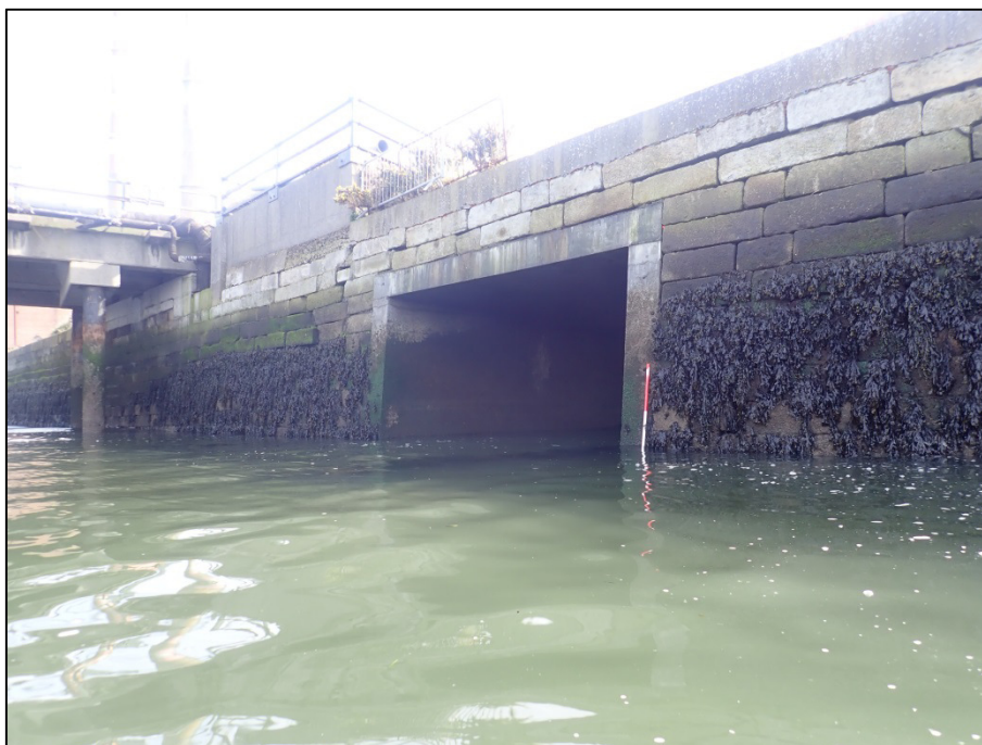
Plate 34: East-southeast facing view of Feature F02 showing impacts to the quay-wall from a box-culvert and the downstream Sludge Jetty (1m scale).
