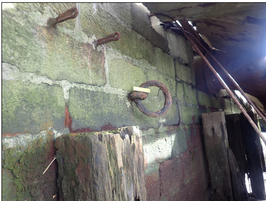
Plate 57: Example of wrought-iron mooring rings that are retained along the façade of masonry quay Feature F03; on east side of harbour basin (150mm scale).
