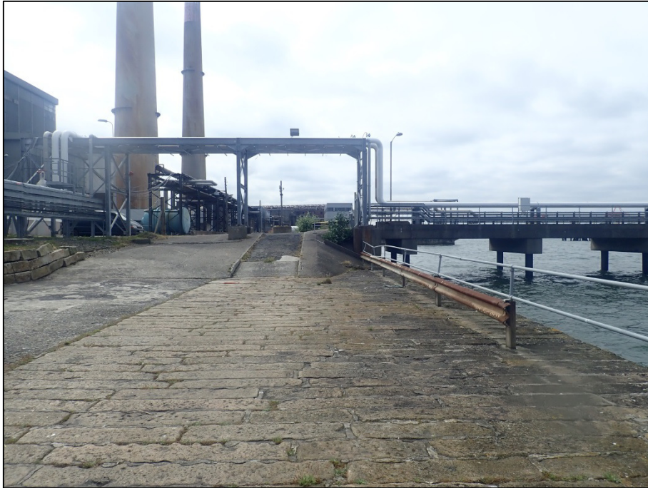
Plate 74: West-facing view of the surface of the sea-wall with NORA Oil Jetty in background; Survey Area 4, GSW-west 3 (1m scale).
