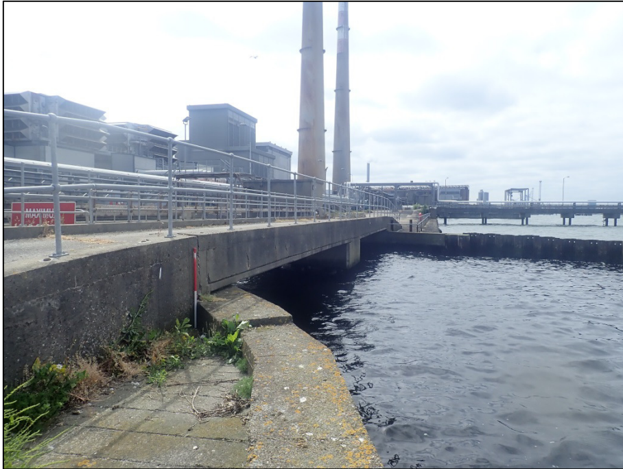
Plate 76: West-facing view of outfall channel that truncates c. 22m section of the GSW between ITM 720820E, 733815N and ITM 720840E, 733518N (1m scale).
