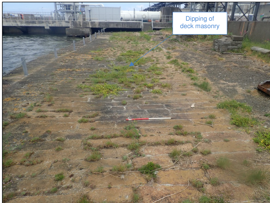
Plate 70: East-facing view of the surface of the sea-wall; Survey Area 4, GSW-west 1 (1m scale).
