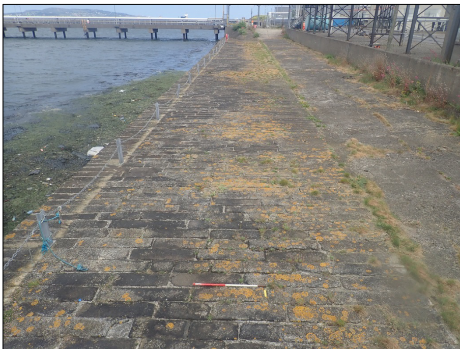
Plate 72: East-facing view of the surface of the sea-wall; Survey Area 4, GSW-west 2 (150mm/1m scales).
