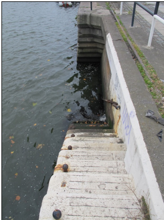
Plate 21: West-facing view of river access steps located immediately upstream of Tom Clarke Bridge.
