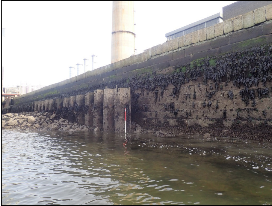
Plate 60: East-facing view of sheet-pile wall and associated rock-armour placed along eastern part of the sea-wall, leading onto the ESB Jetty; Survey Area 4; GSW-West (1m scale).
