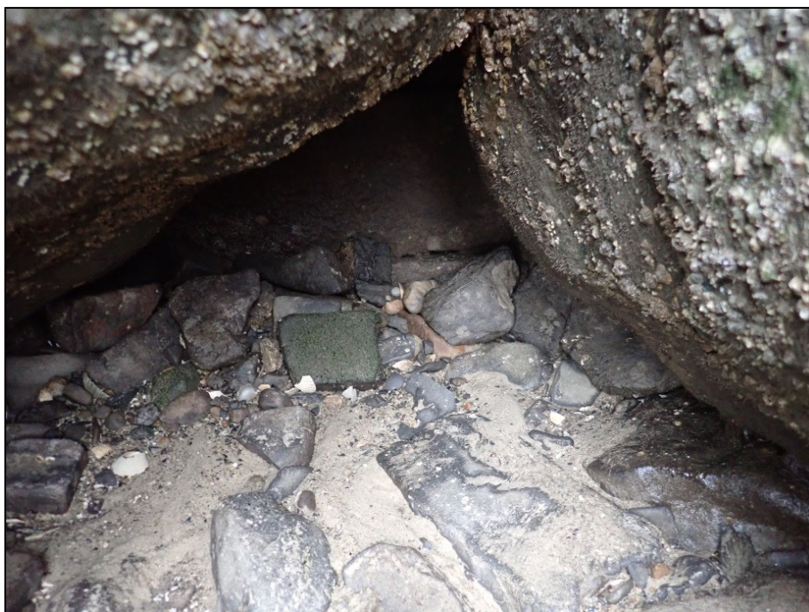
Plate 86: Example shot of large gaps in the rock-armor protection.
