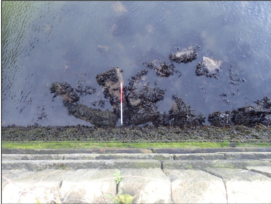
Plate 38: Shot looking down the external façade of the pier-head (Feature F02) showing a stepped profile to the masonry courses (1m scale).
