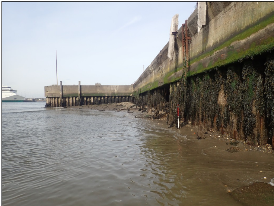
Plate 47: North-facing of sheet pile wall forming a c. 50m-long section of quayside on east side of harbour basin, leading onto modern pier-head at harbour entrance (1m scale).
