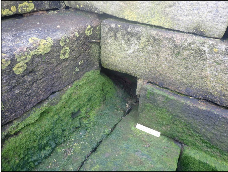
Plate 40: Detail shot showing masonry steps in-set into quay-wall at pier-head, RAS-02 (150mm).
