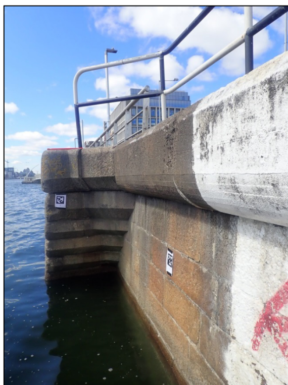
Plate 23: West-facing view of bullnose terminus to cascading masonry on the west side of the upstream river access steps.
