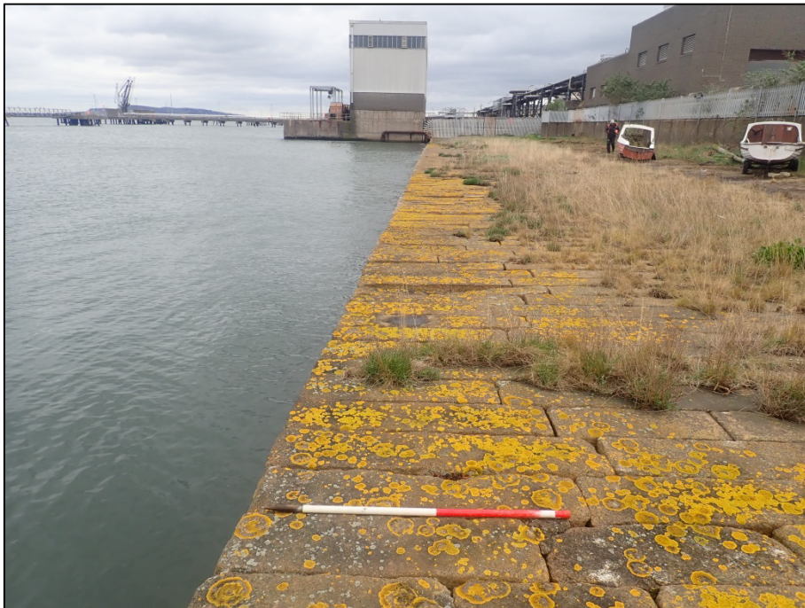
Plate 59: East-facing view along surface of the sea-wall; Survey Area 4, GSW-west (1m scale).
