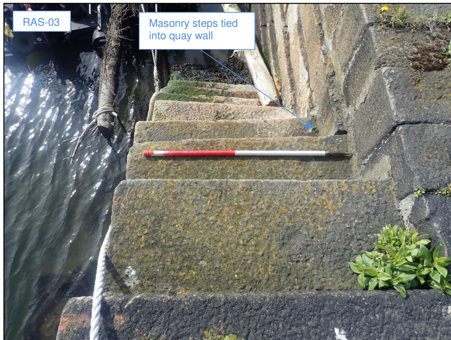
Plate 42: View looking down the set of access steps (RAS-03) located on the south side of the pier-head (1m scale).
