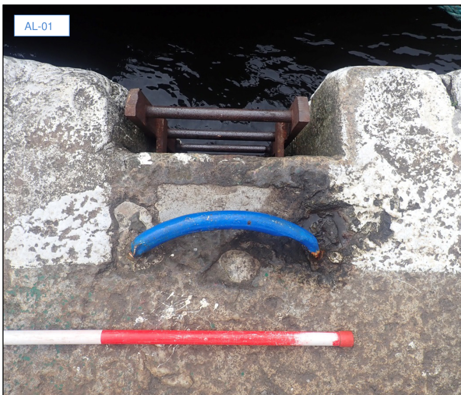
Plate 29: River access ladder and associated grab-handle (AL-01) located at ITM 718051E, 734383N (50mm scale).
