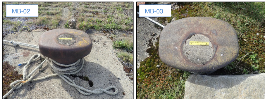
Plate 43: Cast-iron mooring bollards, MB-02 and MB-03, inset into deck of the pier-head of Feature F02 at entrance to Pigeon House Harbour (150mm scale); ITM 720299E, 733844N and ITM 720315E, 733844N respectively.
