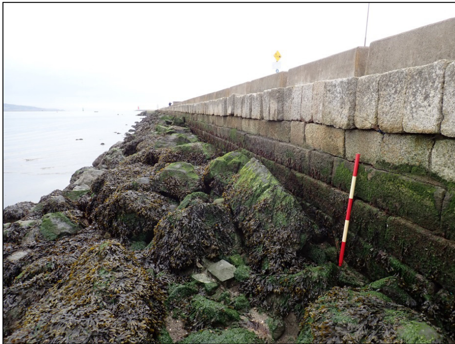
Plate 84: East-facing view of the channel-side façade of the GSW at a point c. 20m east of the ESB Jetty (Survey Area 4, GSW-east); note four masonry courses visible below capping stones before being covered by rock-armour protection (1m scale).
