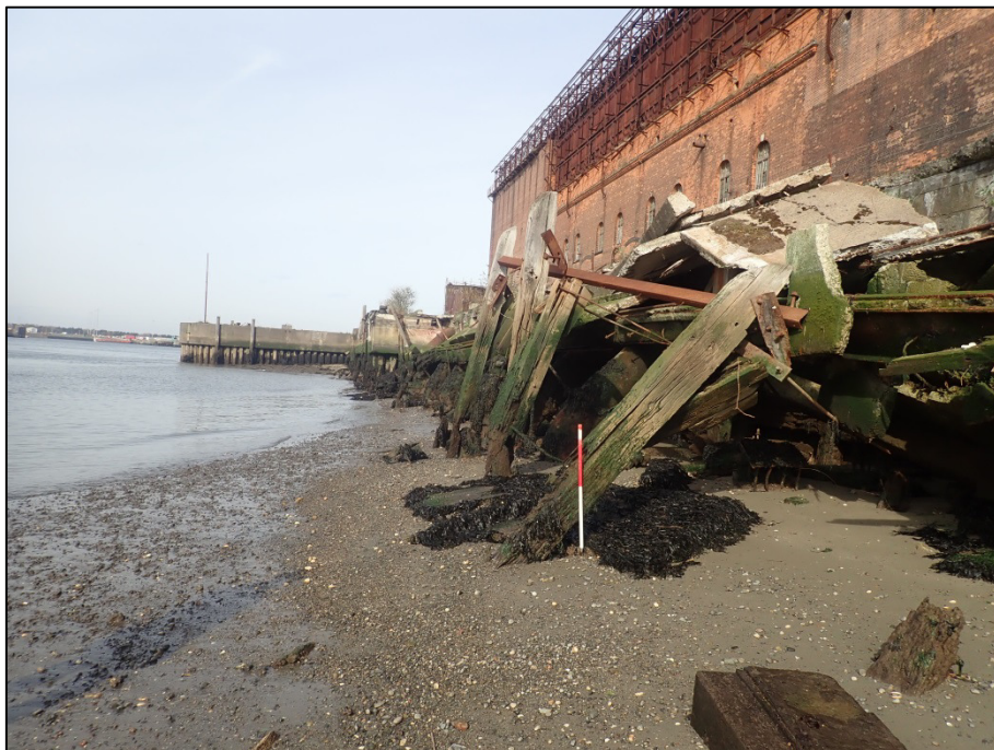
Plate 55: North-facing view of collapsed, twentieth century, quayside on east side of harbour basin, behind which an original masonry quay are located (1m scale).
