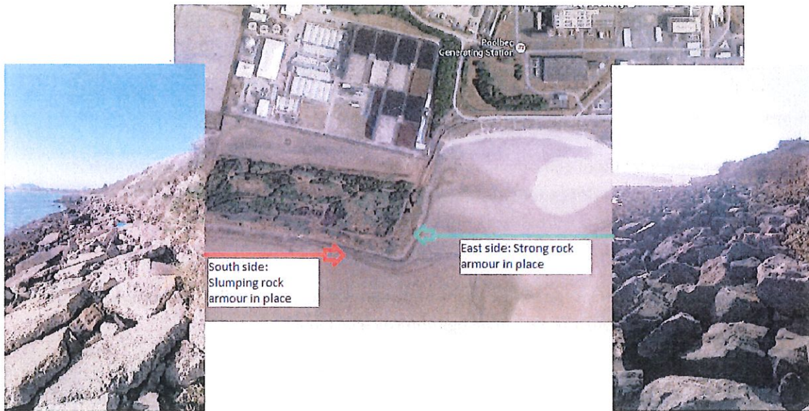
Image 4A, 4B, and 4C: Showing the comparison of rock armour on both the East and South side of the Ringsend site. (Source: Google maps)
