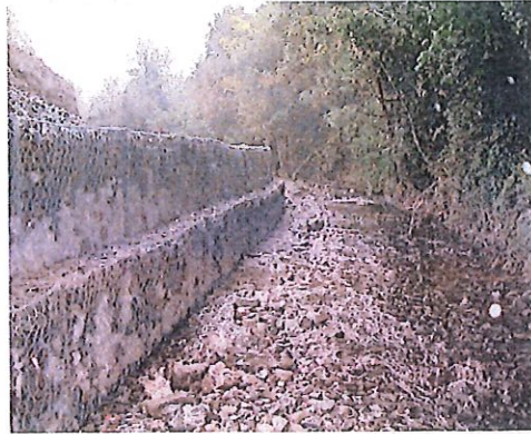
Image 7: Showing an example of woven mesh gabions constructed along a riverbank. (Source: www.geo-coastal.ie )
