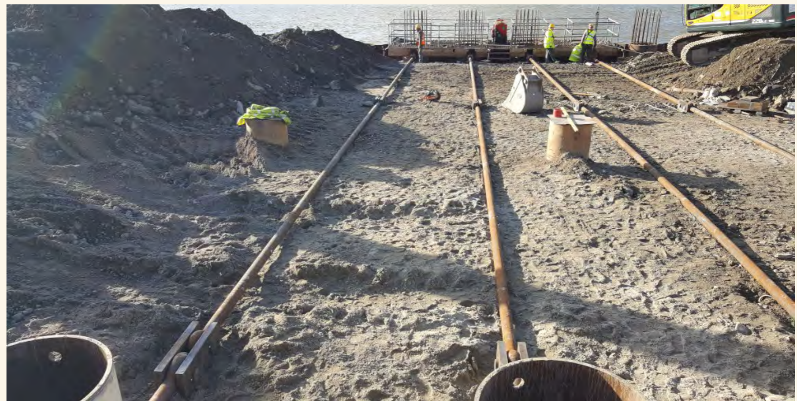
View looking south during the construction of the new quayside for Berth 32, showing the steel tie beams that link the anchor piles (bottom of picture) to the new quayside in the distance Source: ADCO for DPC
