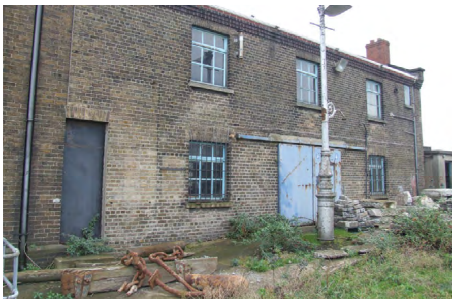
West-facing elevation of Pumphouse No.1 and lamp standard in 2020 prior to rehabilitation works Source: ADCO for DPC
