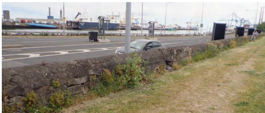
View looking East from York Road along the parapet of the Great South Wall
