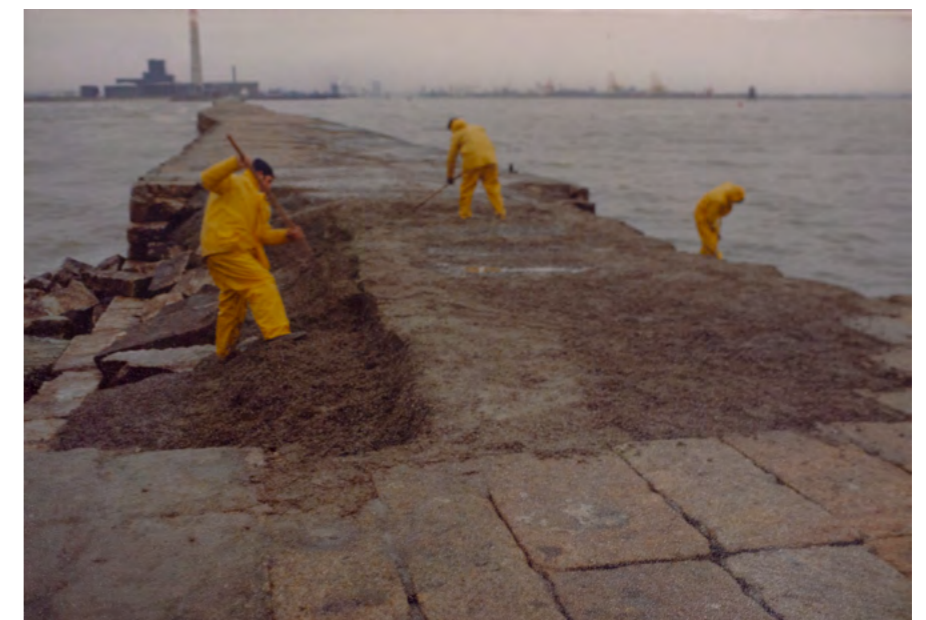
Photograph taken after the storm in 1981, illustrating the damage to the Great South Wall Source: Dublin Port Company, Port Engineer
