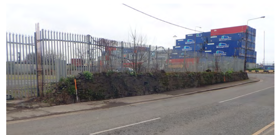
Parapet of the GSW stands today as a low boundary wall on Pigeon House Road in close proximity to the operational port, and has been breached in many places Source: ADCO for DPC
