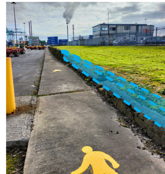
▼ 03. Section of the Great South Wall with segment missing forming a boundary to John Nolan Transport on Pigeon House Road
