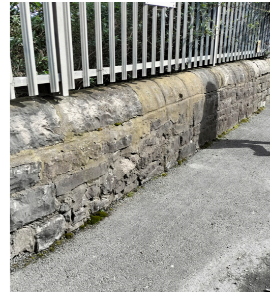
▲ 04. Section of the Great South Wall forming a boundary to Ringsend Waste Water Treatment Plant on Pigeon House Road
