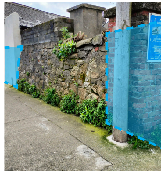
— Great South Wall Missing Portions
