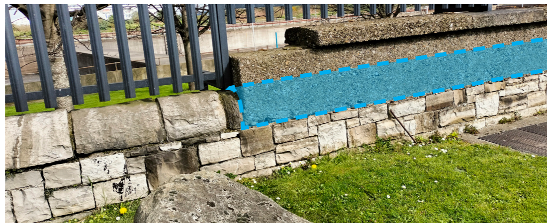
Great South Wall Missing Portions
