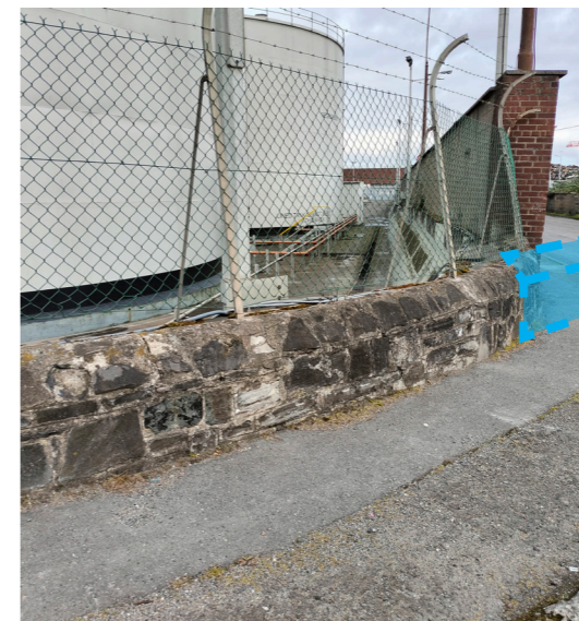
▲ 06. Section of the Great South Wall forming a boundary to the entrance of Hammond Lane Metal Recycling with segment missing on Pigeon House Road
