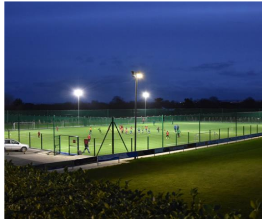
Sportslite 12 600W IP66 mounted on 12-meter poles - Location: Port Park
